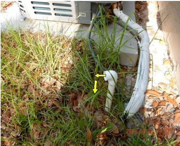
Condensate Line: Exposed to misc. particles in the air.
