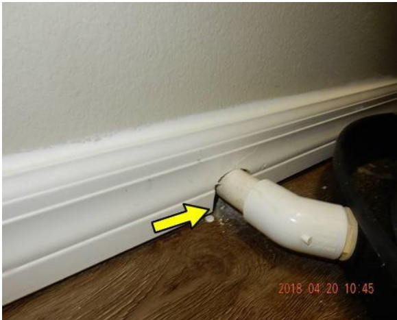
Baseboard: Visible gap.
