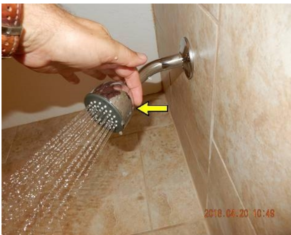
Main Bathroom - Shower Head: Visible, minor leak.
